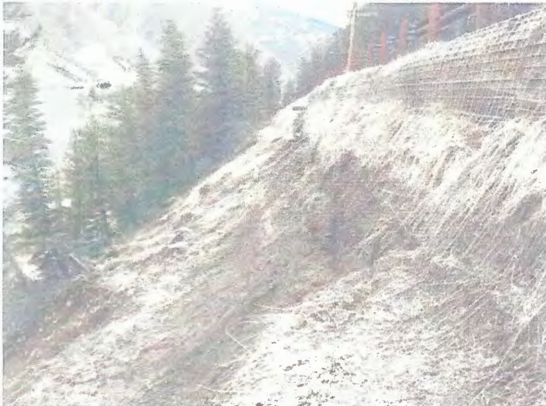
Existing Hilfiker Wall and Slope Condition from STA 1+20 (Wall Toe) Looking Northwest – April 10, 2017
